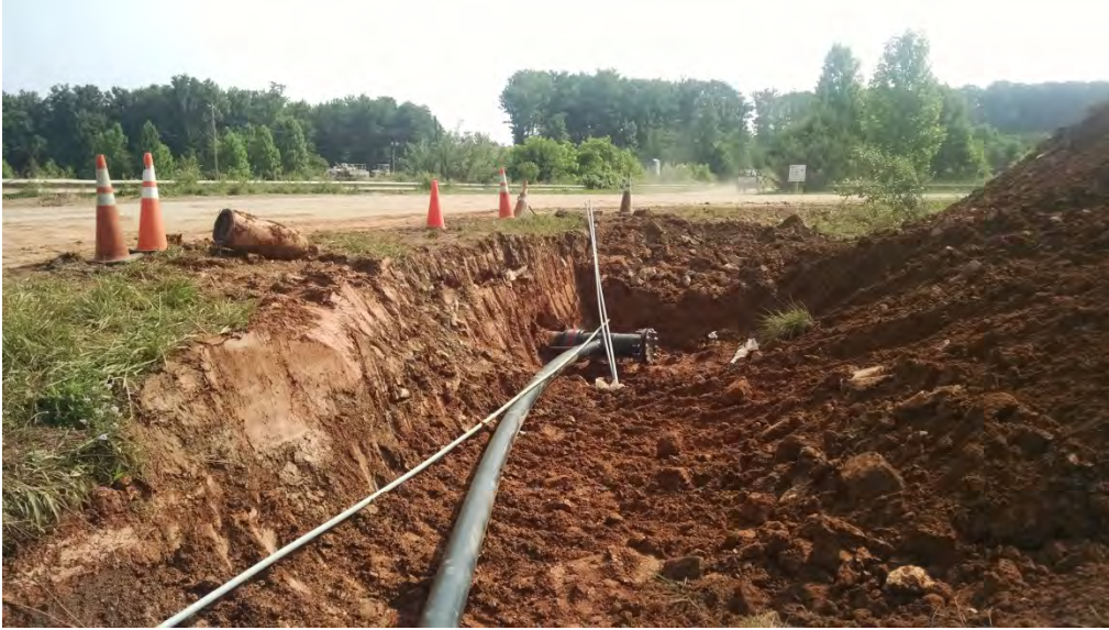
90 degree tee immediately before the road crossing, accomplished with an electrofusion coupling. Note the blind flange allowing for future expansion to the south (6/11/15).
