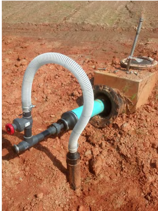
Example of leachate cleanout utilizing Waste Management-style wellhead for connection to LFG collection system (6/23/15). Eight total leachate cleanouts were connected to vacuum.
