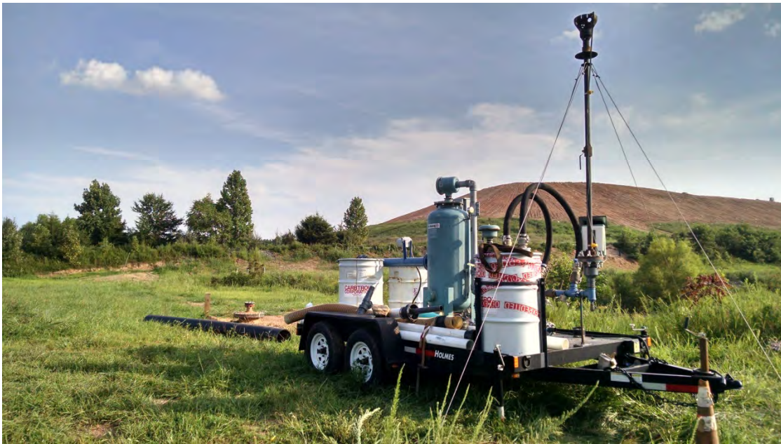
Mobile blower station and temporary SCS-rental flare setup (8/17/15).
