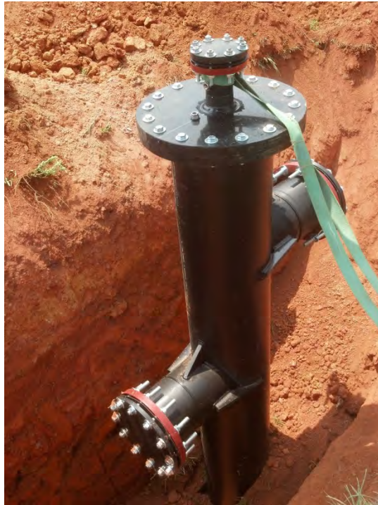
10-foot deep by 18-inch diameter sump installed across road near northeast corner of the landfill (6/11/15).
