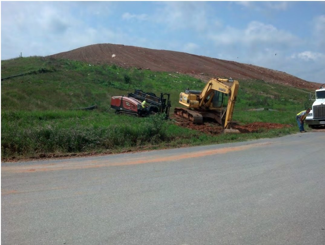
Horizontal directional drilling by Toney Construction. The borehole was for the 12" header under the paved access road at the northeast corner of the landfill (6/8/15).
