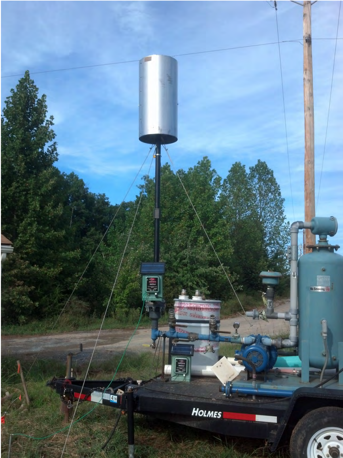
Mobile blower station and Authority-owned flare setup, installed 9/23/15. The flare is a CF-10 Solar Spark flare with a crown ring and heat shield to promote combustion and minimize emissions.
