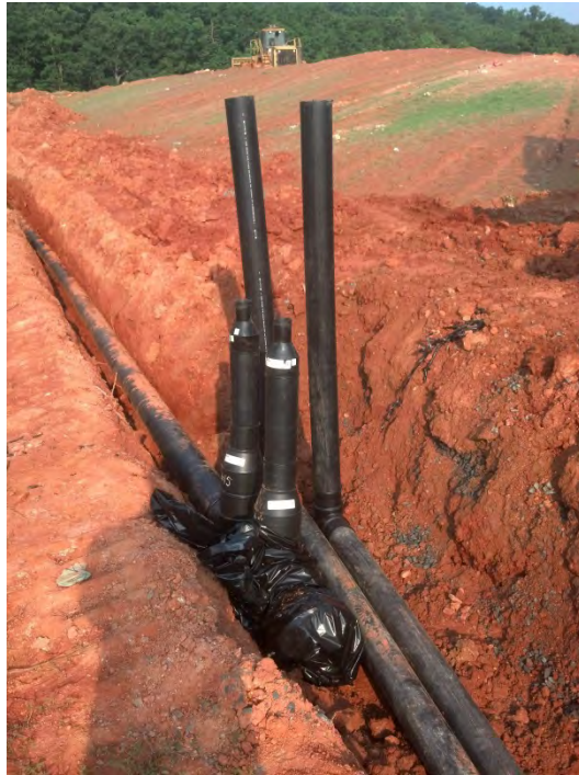
Stub-ups for remote wellheads located near the southwest corner of the landfill (6/11/15).
