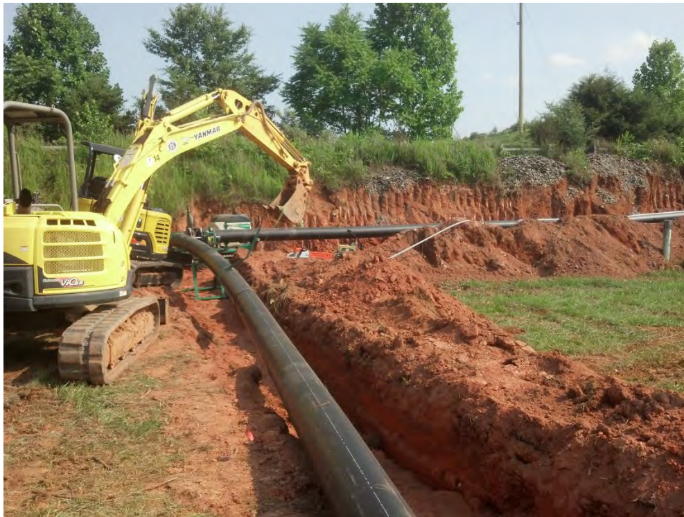
90 degree bend immediately after the road crossing, leading to condensate manhole and blower/flare station. The 90 was accomplished with a butt-fusion weld (6/11/15).
