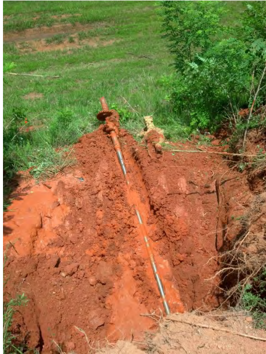
Horizontal directional drill bit surfacing from underneath paved haul road. The borehole was lubricated with water prior to header pipe being pulled through (6/8/15).
