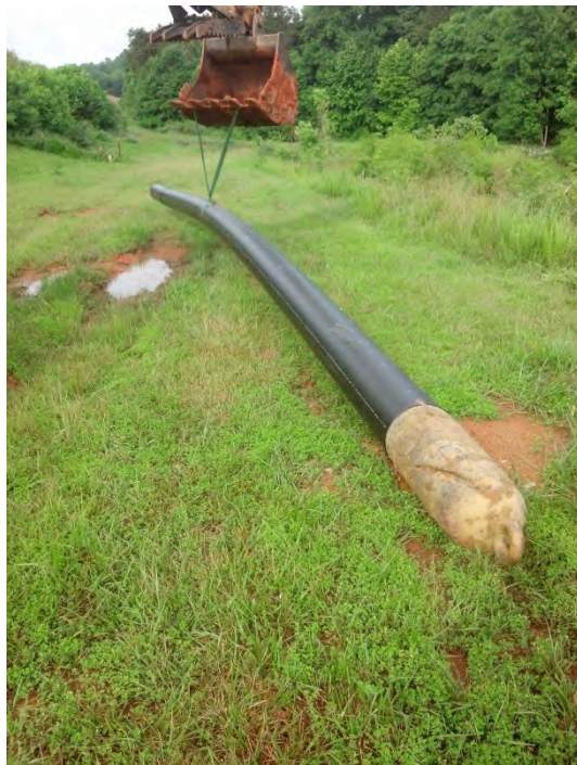
12-inch HDPE header pipe prior to being pulled through the horizontal borehole underneath the access road. As shown the pullhead (cap with pull loop) was fused onto the pipe (6/8/15).
